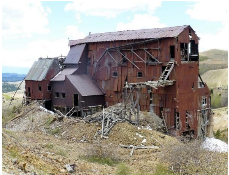
Figure 4. The Vindicator ore sorting house is one of the best-preserved buildings of its kind in the mining district. Photo © by S. W. Veatch.
